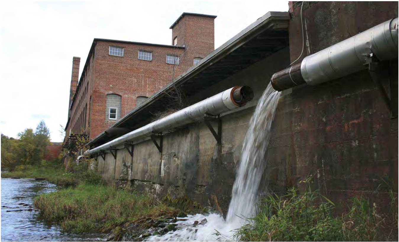
The broken pipe that runs from Laurel Lake to the Eagle Mill is one of two sources of zebra mussels to the Housatonic River.
